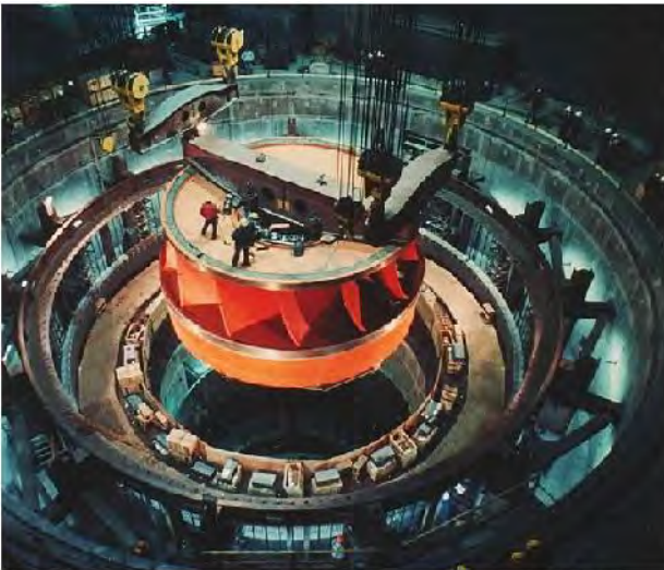
A Francis turbine runner, rated at nearly one million hp (750 MW), being installed at the Grand Coulee Dam, United States.
